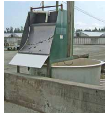
LAMINAR FILTER – PERMITS WATER REUSE IN BLOCKWASHING.
