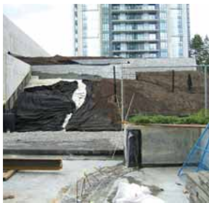
Figure 5. Filter fabric is drawn over the drainage layer and covered with growing medium.
